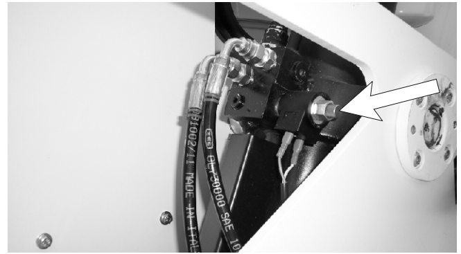
Figure 7.21.1 - Emergency Lower Valve, Controlling Lower Boom
