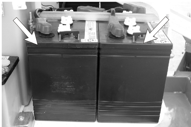
Figure 11.6 - Two DC Motor Batteries (Petrol/Diesel Engine Side)
