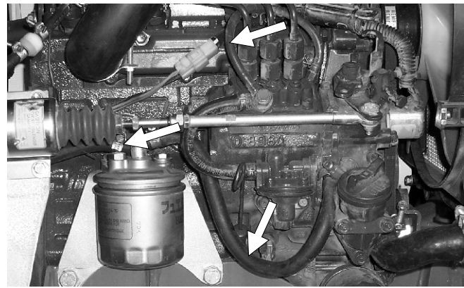
Figure 7.4 - Fuel Leaks in Hoses & Joints
