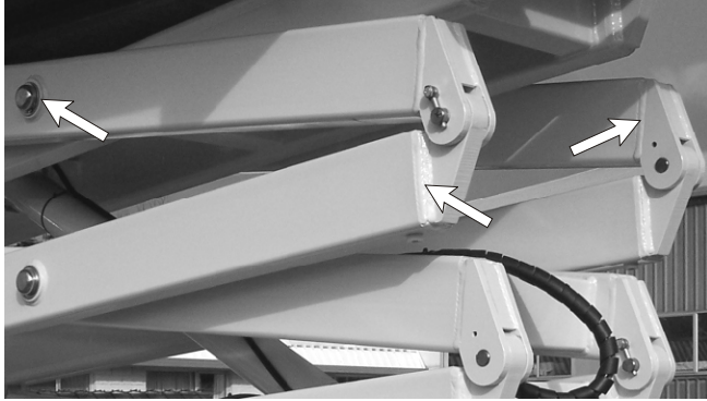
Figure 7.19 - Structural Damage and Welds
