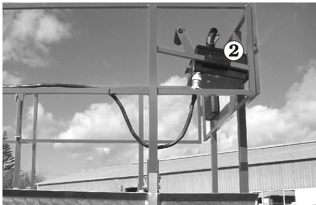
Figure 6.1.2 - Control Box Location, Platform Position
