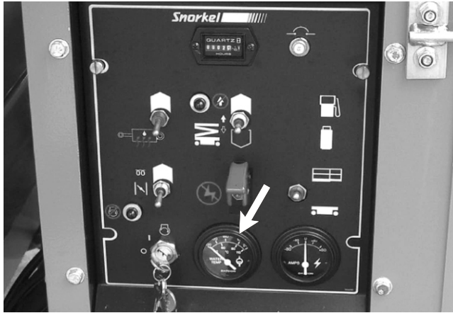
Figure 4.1 - Water Temperature Gauge
